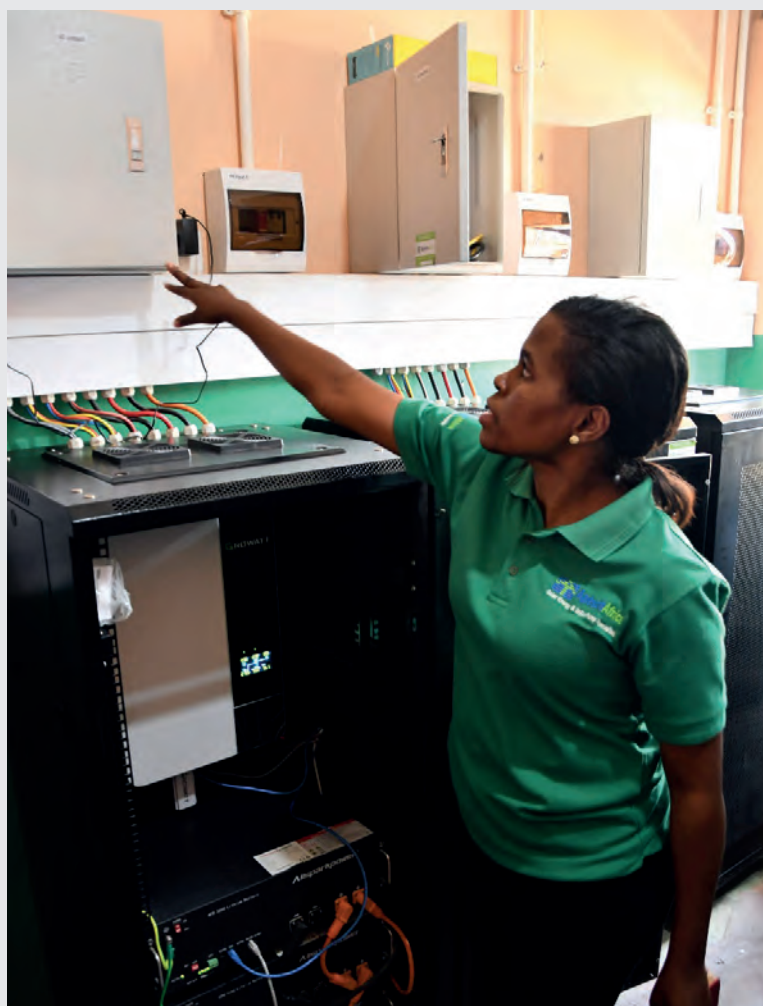
Solar infrastructure installed at Bukomero Health Center IV
